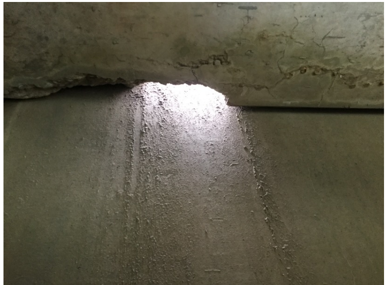
Damage to left bank panel
