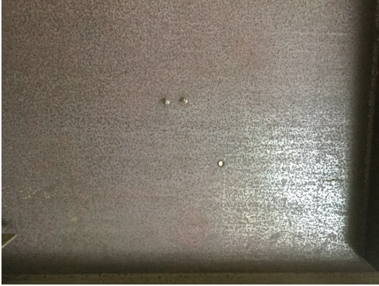
Downstream web damage
