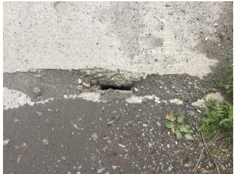
Damage to left bank ballast wall and deck panel
