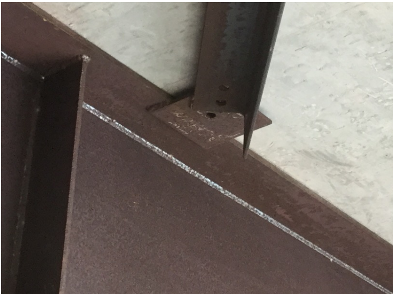
Bracing that was planned for bolts was welded 1 end
