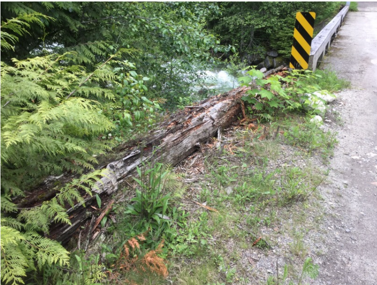
Fender log condition
