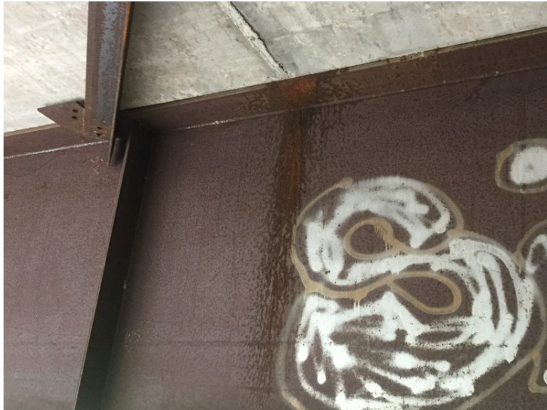
Indications of water getting through deck joints
