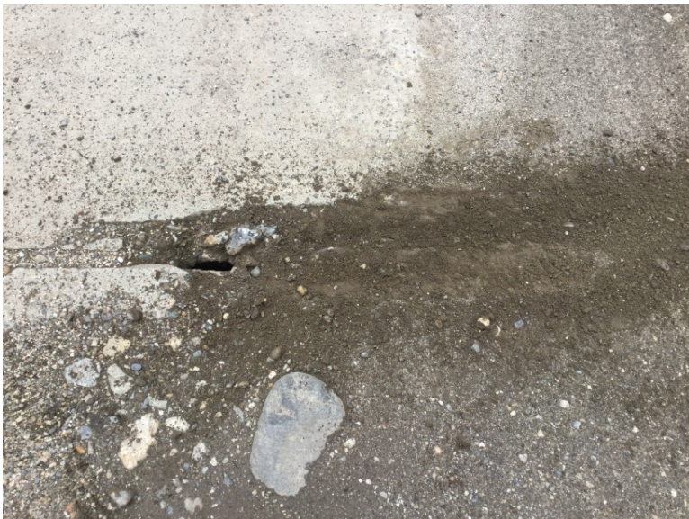
Damage to right bank ballast wall and deck panel
