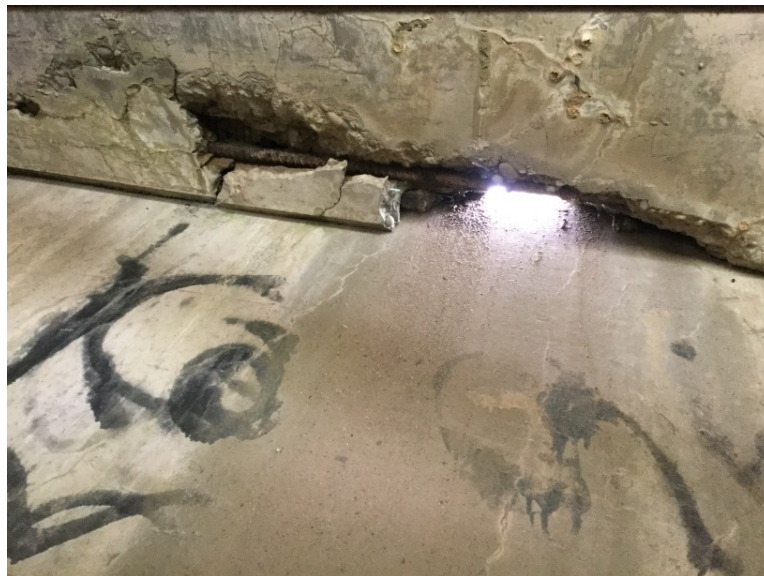
Damaged panel at right bank
