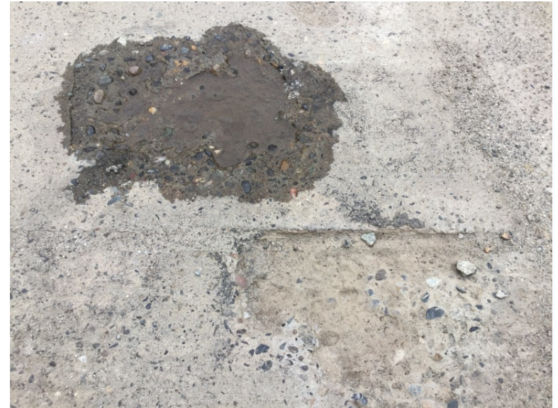
Damage to deck panels on surface
